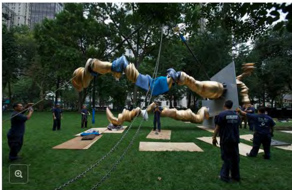
Workers for Dun-Rite Specialized Carriers orchestrated the placement of "Points of View" in Madison Square Park on Friday. Benjamin Norman for The New York Times
